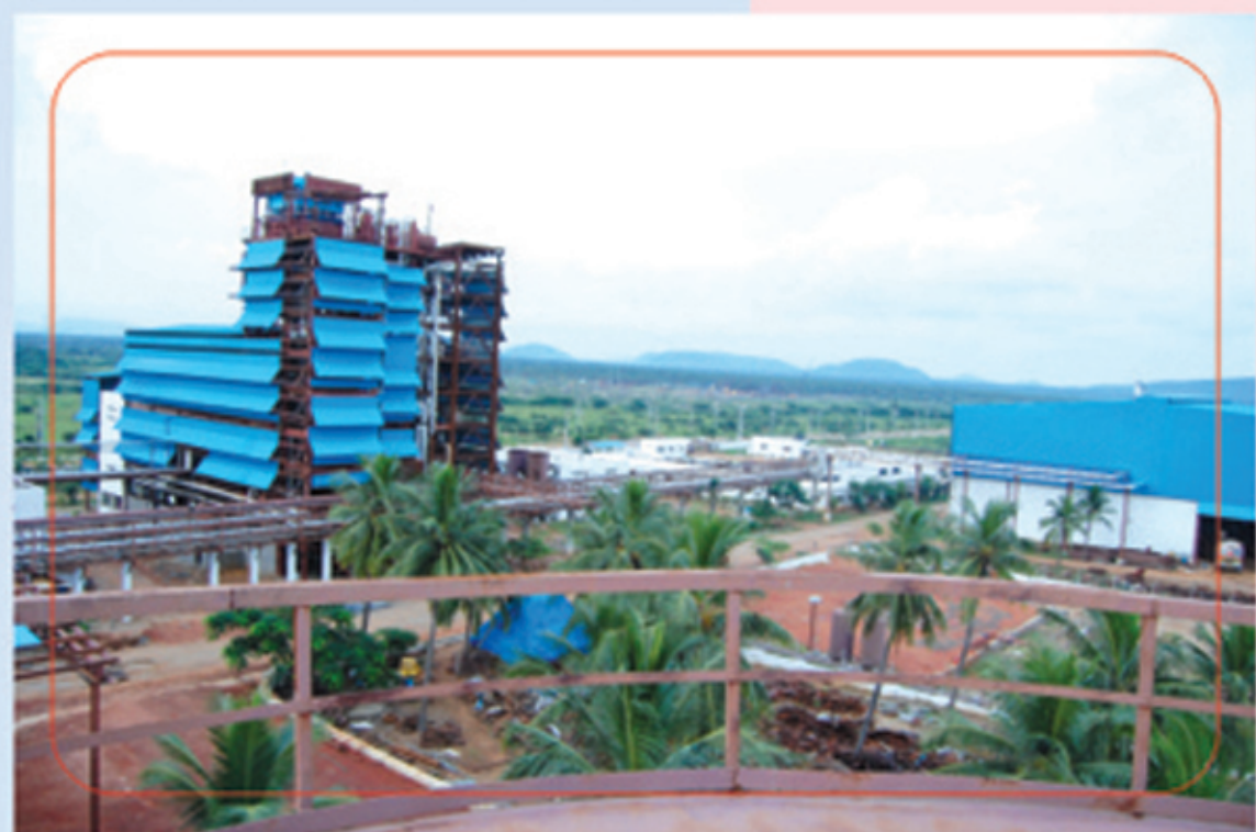
SBT Biodiesel Plant - Visakhapatnam
